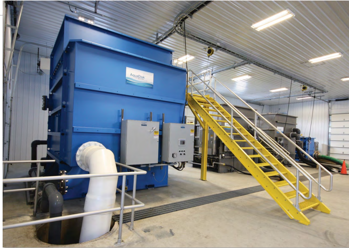
First Aqua MegaDisk® prototype installed at R&T Center
