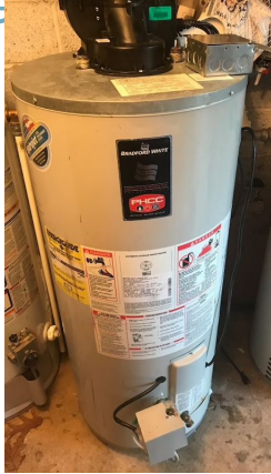
Hot water heating
